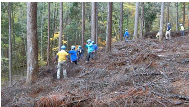
Site preparation: working by hand to gather up branches and foliage scattered on the ground
