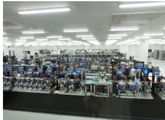
Clean room with latest air-conditioning system
