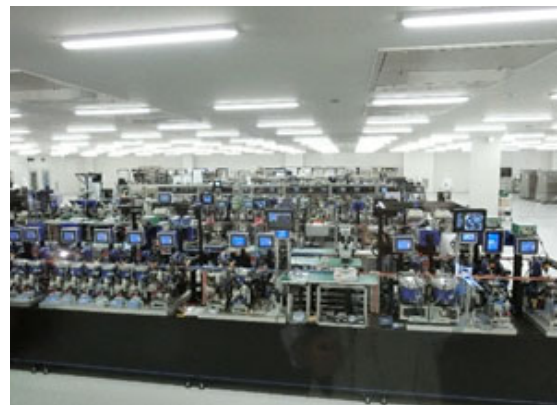
Clean room with latest air-conditioning system
