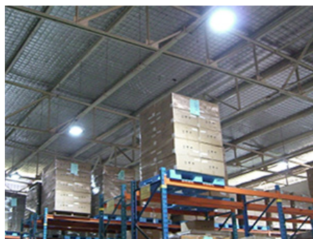
Daytime warehouse lighting
