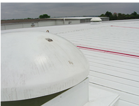
Electric rooftop exhaust fans for heat discharge
