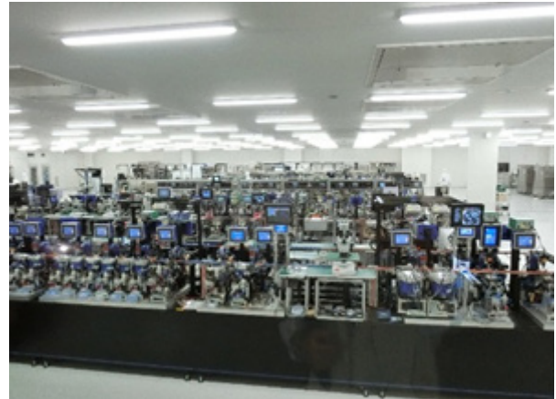
Clean room with latest air-conditioning system
