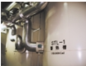
Thermal storage air-conditioning equipment at the Hatsudai Head Office utilizes cold water created using electric power at night to reduce electric power consumption during the day.
