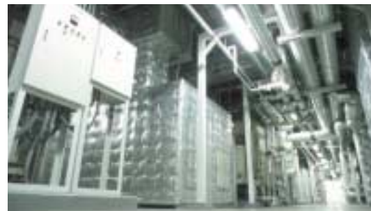
Air-conditioning facilities of Kochi Casio
