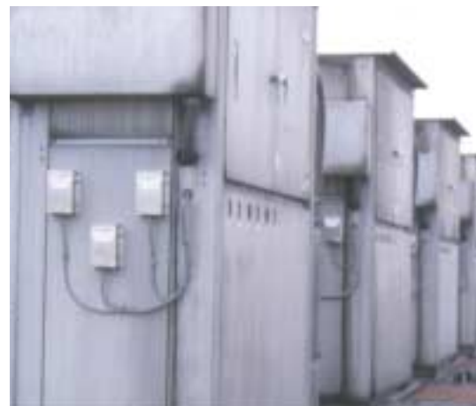
Casio Electronic Manufacturing's cooling towers equipped with new control system
