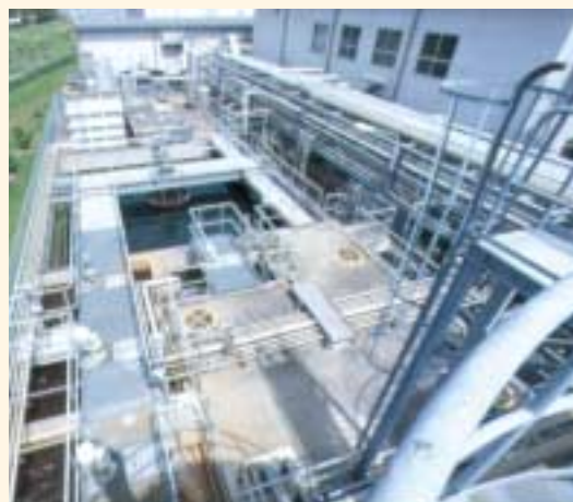
The water treatment facility at Kochi Casio
